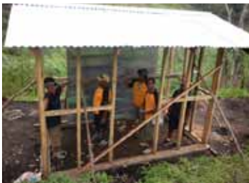
KTA chairman Mr Ruben Maleva (centre rear), Deputy Chairman and landowner rep Mr Robert Batia (second from left) inspecting the construction during their 2013 KTA Management Trek.
