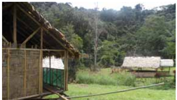
The picture of this house shows traditional building materials decaying
